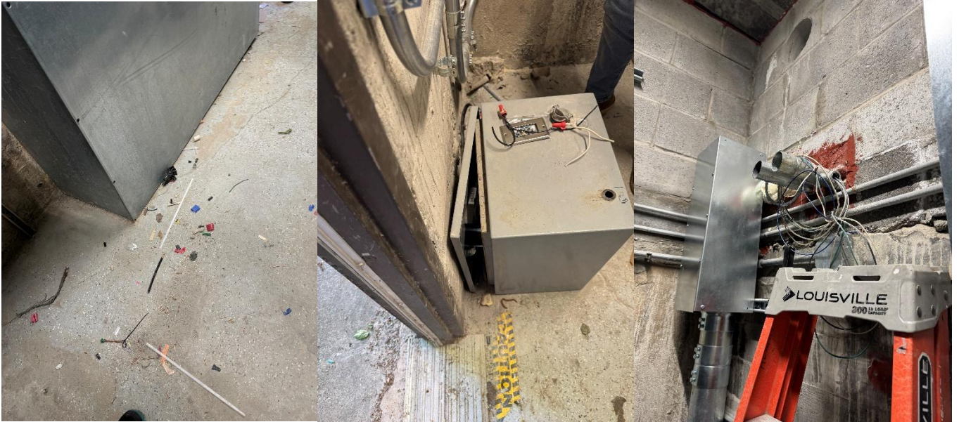
Figure 3: Elec 120: General Cleanup Issues in Space
