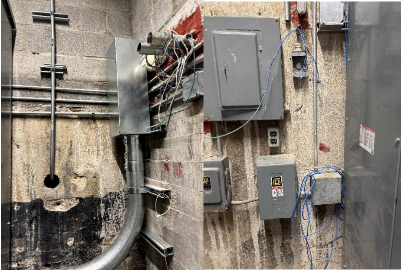
Figure 1: Conduit Penetrations in Electrical Vault Require Patching/Capping, Terminate conductors, Support Conductors
